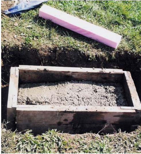
On left, a new base partially filled with concrete and foam setting form in background.
